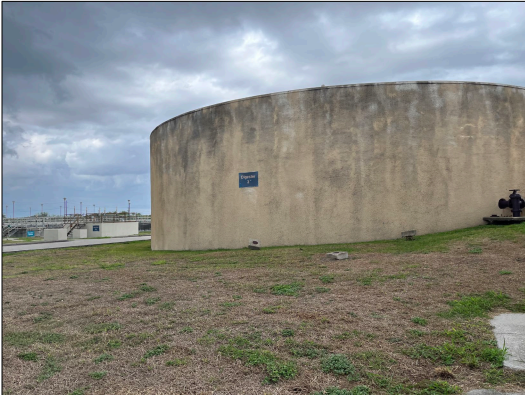
53. Photo taken from east side of WWTP facing southwest. A primary digester labeled "Digester 3" can be seen.
