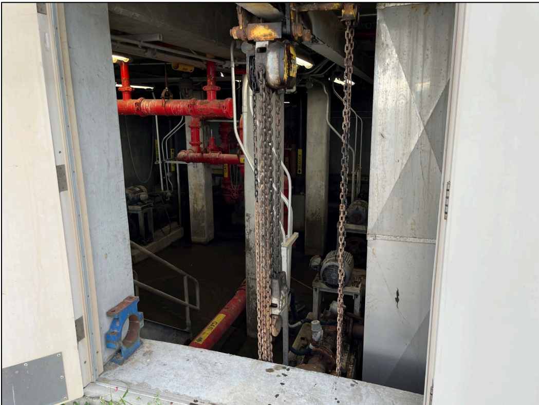
52. The interior of the digester pump building can be seen. Piping, cranes, and other equipment can be seen.
