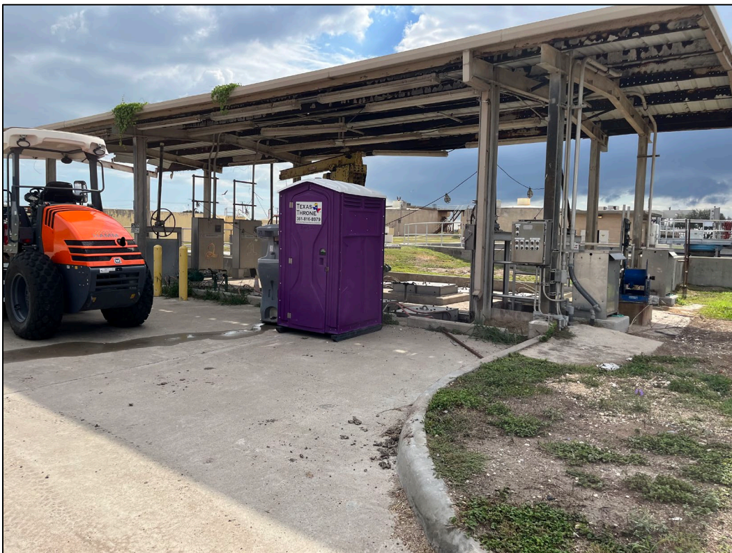
18. Photo taken on west side of WWTP facing northwest. A portable toilet and a small roller/compactor can be seen near the out-of-use UV disinfection treatment unit.
