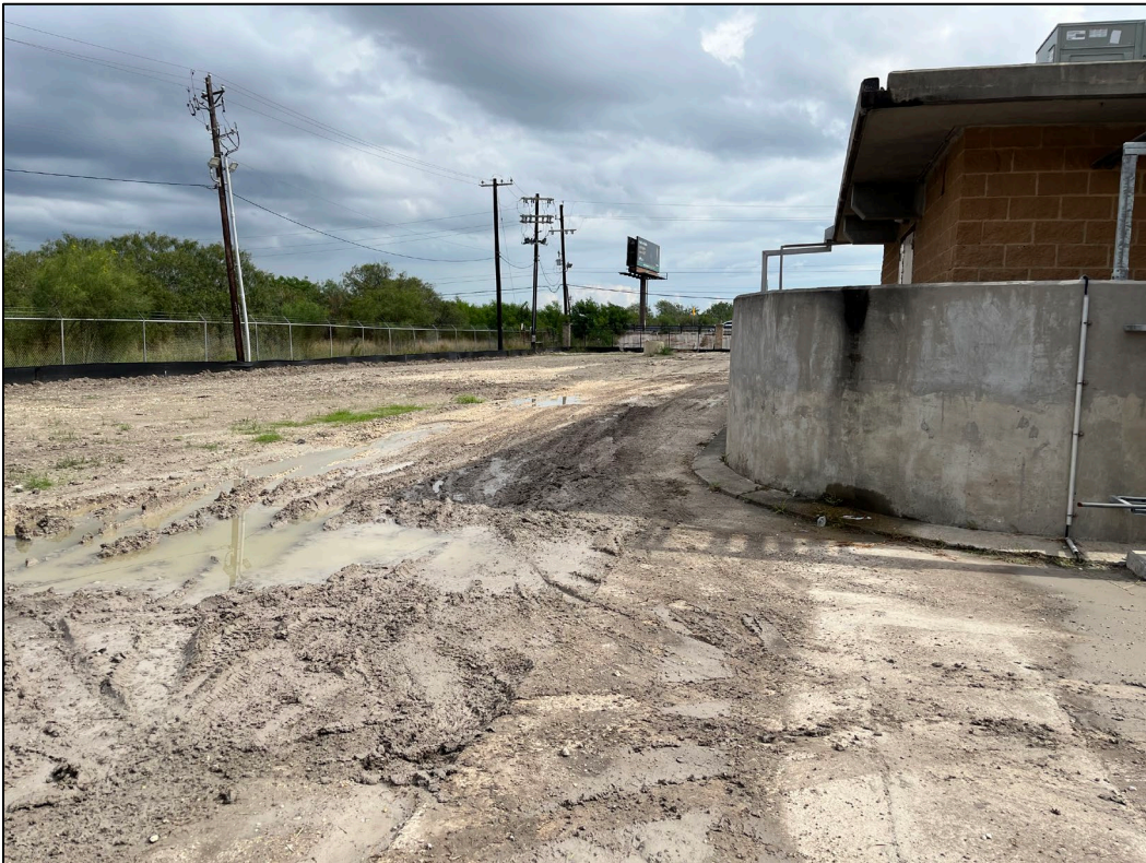
28. Photo taken from west side of WWTP facing north. The northwest corner of the subject property can be seen. The control room is visible to the right.
