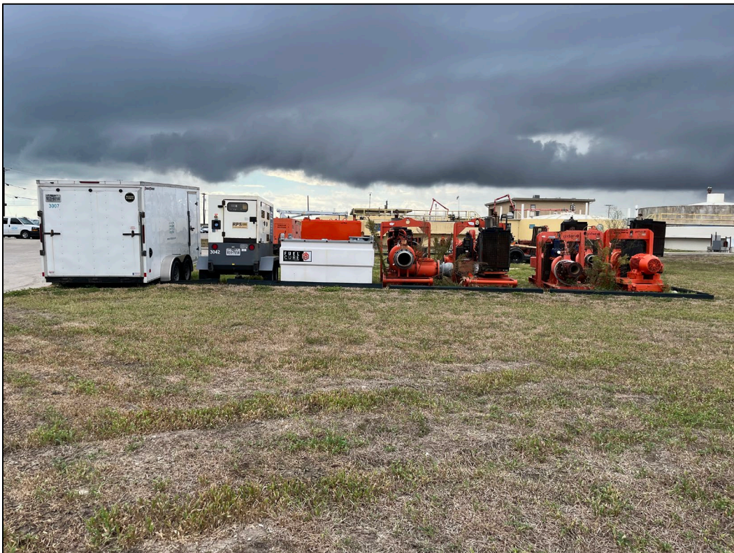
34. Photo taken in north-central portion of the WWTP facing east. A storage area with a trailer, portable diesel power system, fuel storage containers, and spare pumps can be seen.
