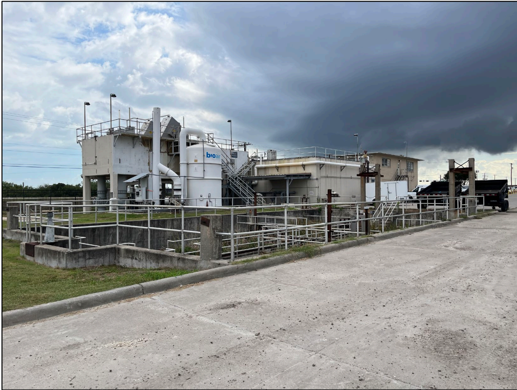
33. Photo taken in northwest portion of WWTP facing northeast. The WWTP influent structure can be seen.
