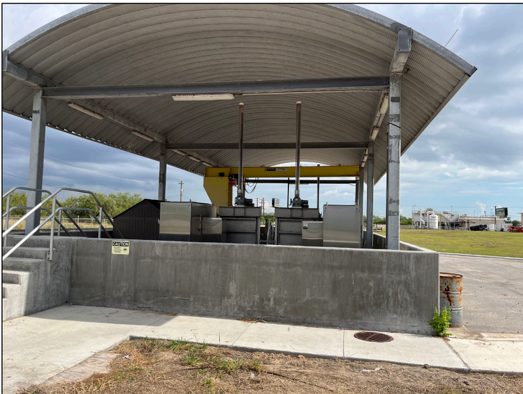
24. Photo taken from west side of WWTP facing north. The south end of the UV system facility can be seen. On the right side of the facility, a drum can be seen.
