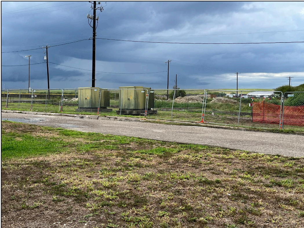
12. Two pad mounted transformers can be seen on the south portion of the subject property near the sludge drying beds. No markings were observed to indicate the units are PCB-free.
