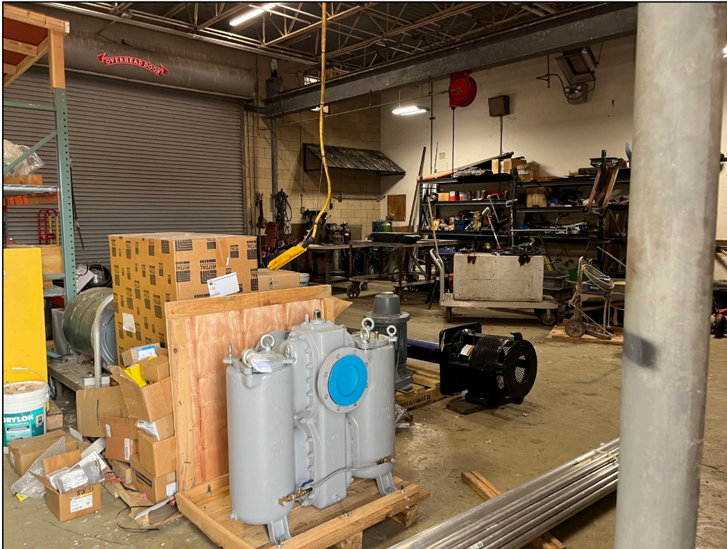
43. Photo taken in northeast portion of WWTP. A workshop and storage area can be seen inside the maintenance building.
