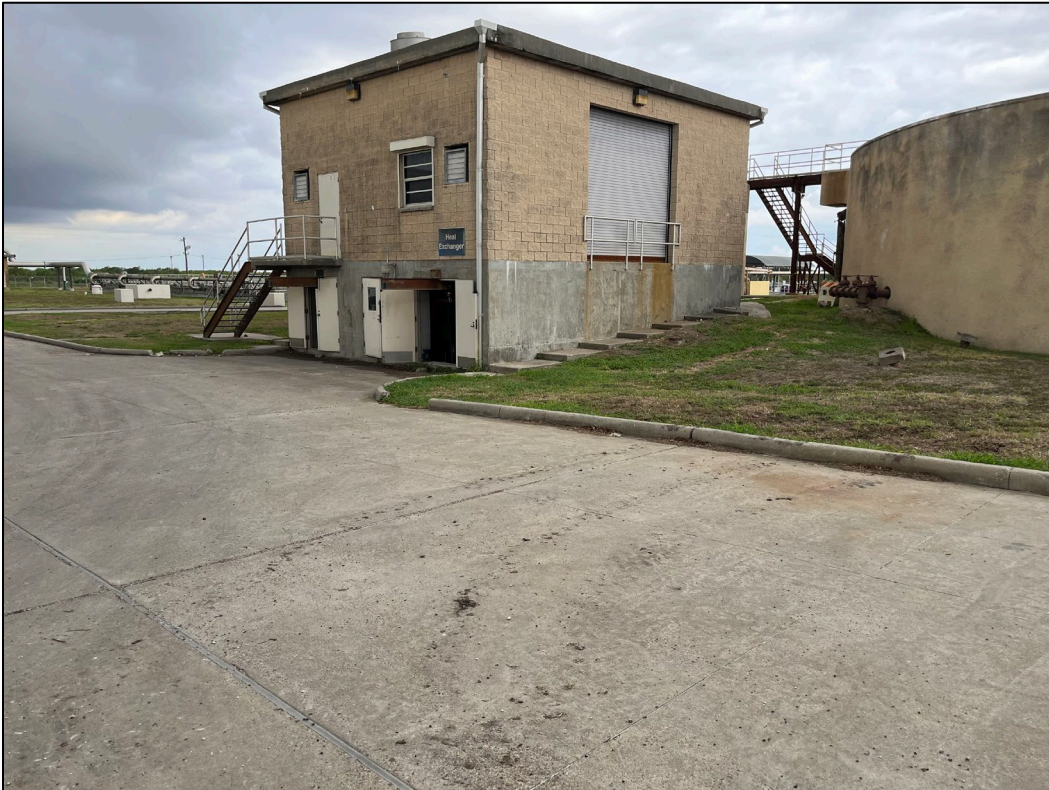
51. Photo taken from east side of WWTP facing west. The digester pump building is shown. A sign stating "Heat Exchanger" is visible.
