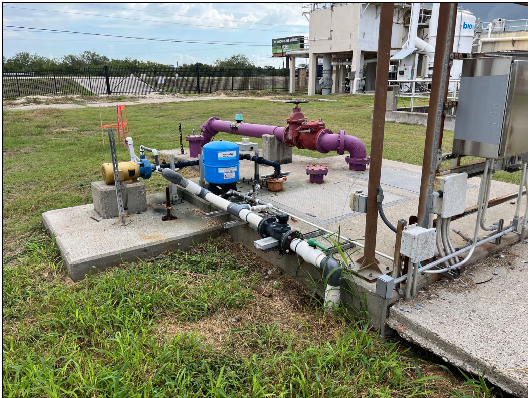
32. Photo taken in northwest portion of WWTP facing northeast. An effluent pump station can be seen.
