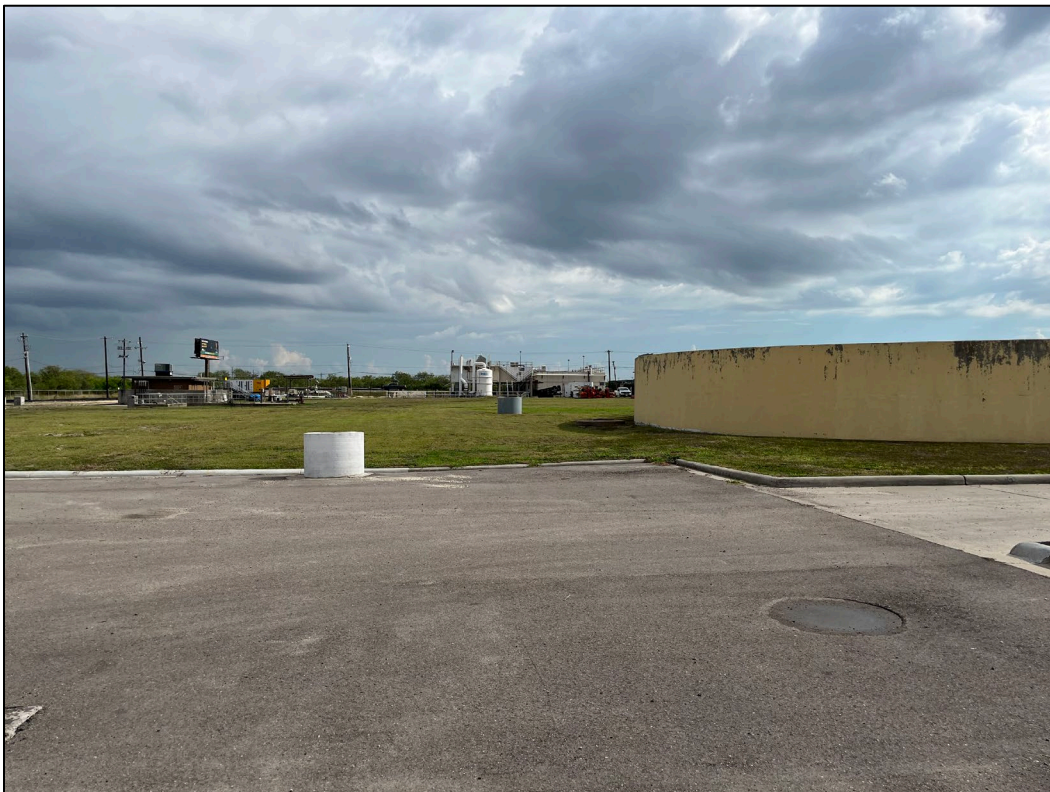
22. Photo taken from west side of WWTP facing northeast. To the right, a primary clarifier can be seen. To the left, an open area, effluent pump structure, and control room are visible. In the center, the influent structure can be seen.
