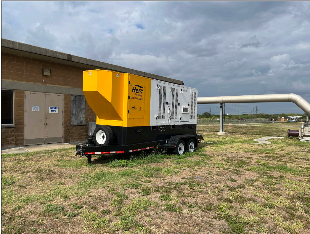
7. Photo taken on east side of WWTP facing west. An emergency generator can be seen near the blower building.
