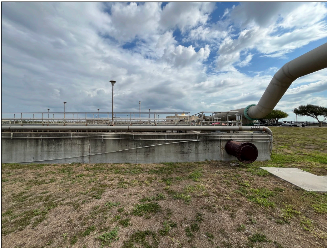
8. Photo taken on east side of WWTP facing north. The south side of the aeration basins can be seen.
