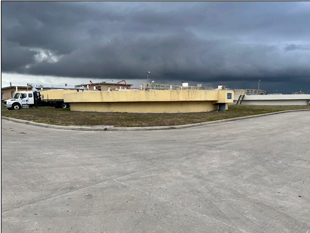
41. Photo taken in north-central portion of the WWTP facing southeast. Primary clarifiers can be seen.
