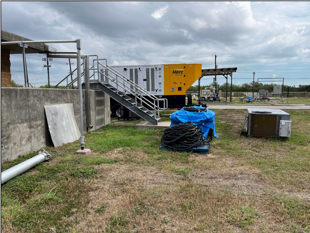
29. Photo taken from west side of WWTP facing north. An emergency generator can be seen near the control room.
