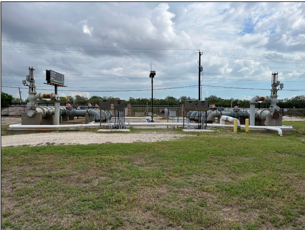
30. Photo taken in northwest portion of WWTP facing northeast. The lift station can be seen.
