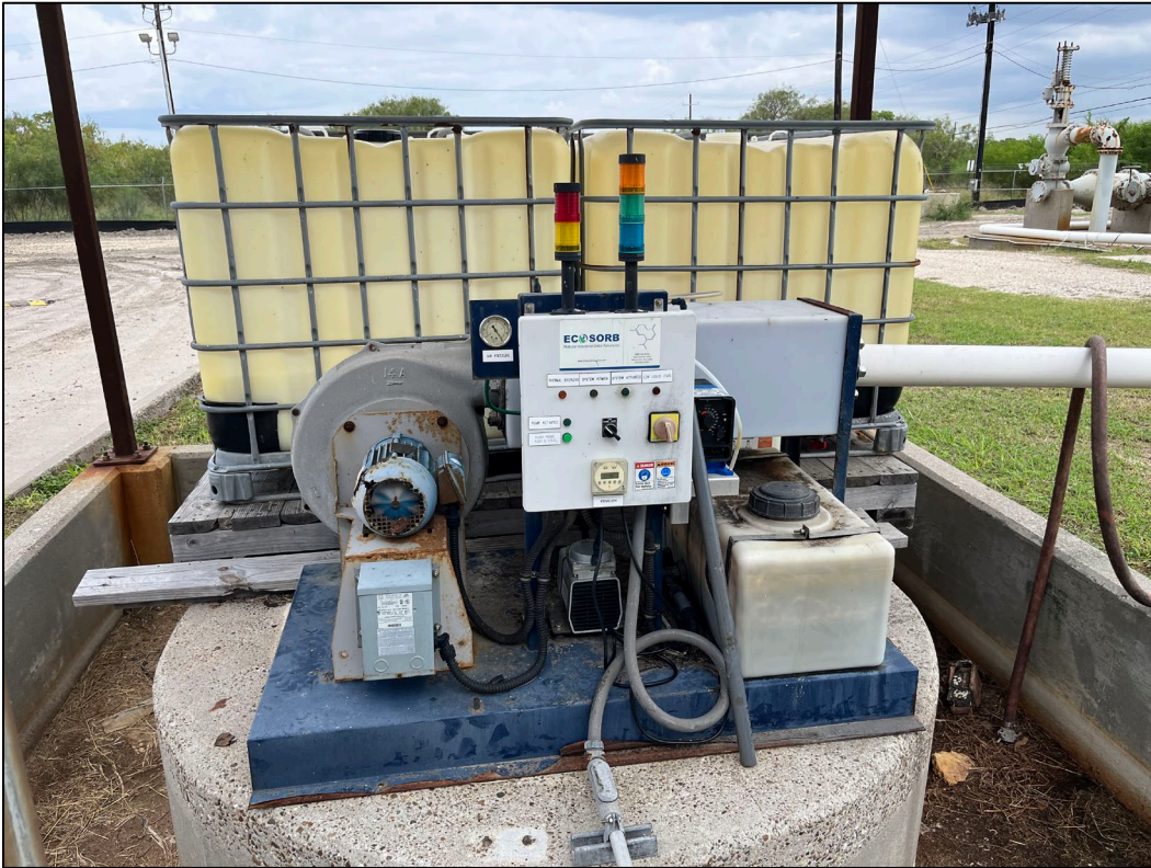
31. Photo taken in northwest portion of WWTP facing northwest. An odor control system can be seen.
