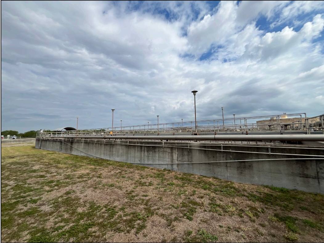
9. Photo taken on the east side of the WWTP facing northwest. The south side of the aeration basins can be seen.
