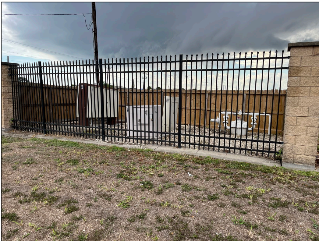
44. Photo taken in northeast portion of the WWTP facing east. A secure area with three underground AT&T cables and a residential gas meter can be seen.
