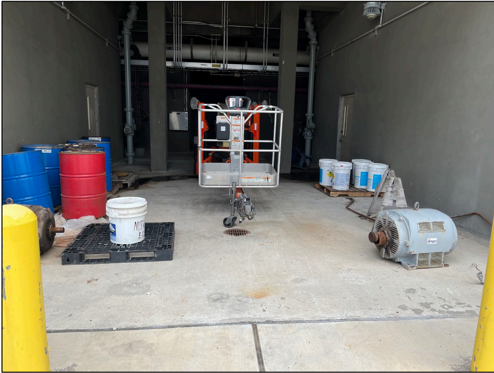
23. Photo taken on north side of the headworks facility on the east side of the subject property facing southwest. A concrete bay being used for chemical storage can be seen. A floor drain that drains back to the wastewater system is visible.
