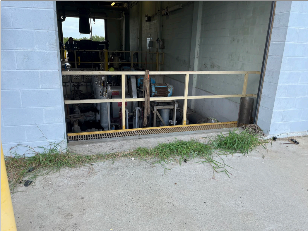
43. Photo taken near Solid Dewatering Facility in northwest portion of the subject property. Equipment in the dewatering facility can be seen.
