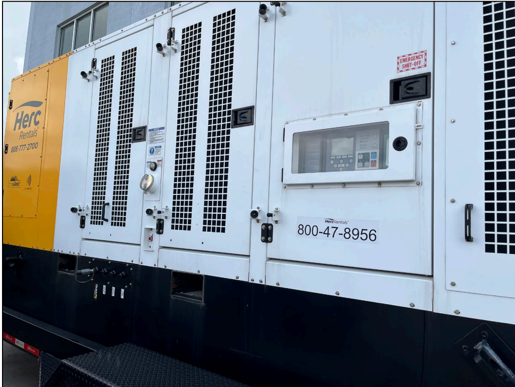
41. Labels on the generator from the previous photo are visible. Labels show that the generator holds 550 gallons of ultra low sulfur diesel fuel when gauge reads full.
