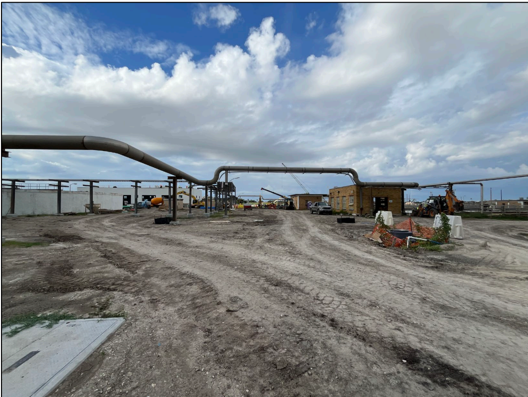
28. Photo taken west of the odor control unit on the east side of the subject property facing southwest. Elevated facility piping, two abandoned blower house buildings, and an out of service aerated sludge holding tank can be seen.
