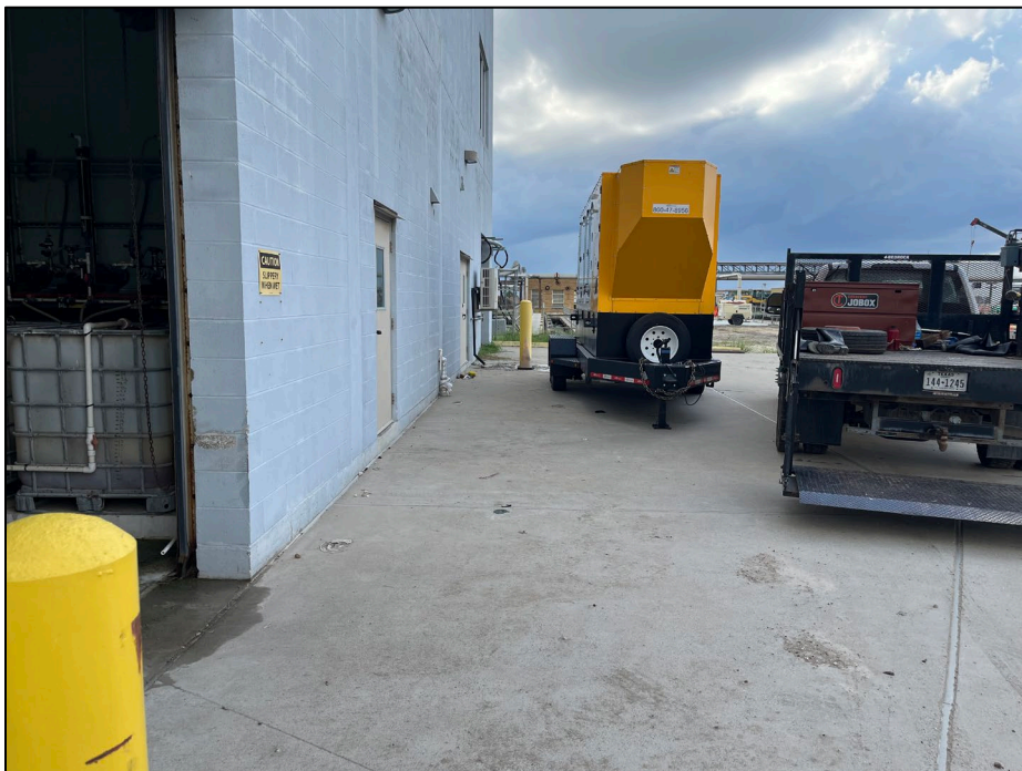
40. Photo taken near Solid Dewatering Facility in northwest portion of the subject property. An emergency generator can be seen.
