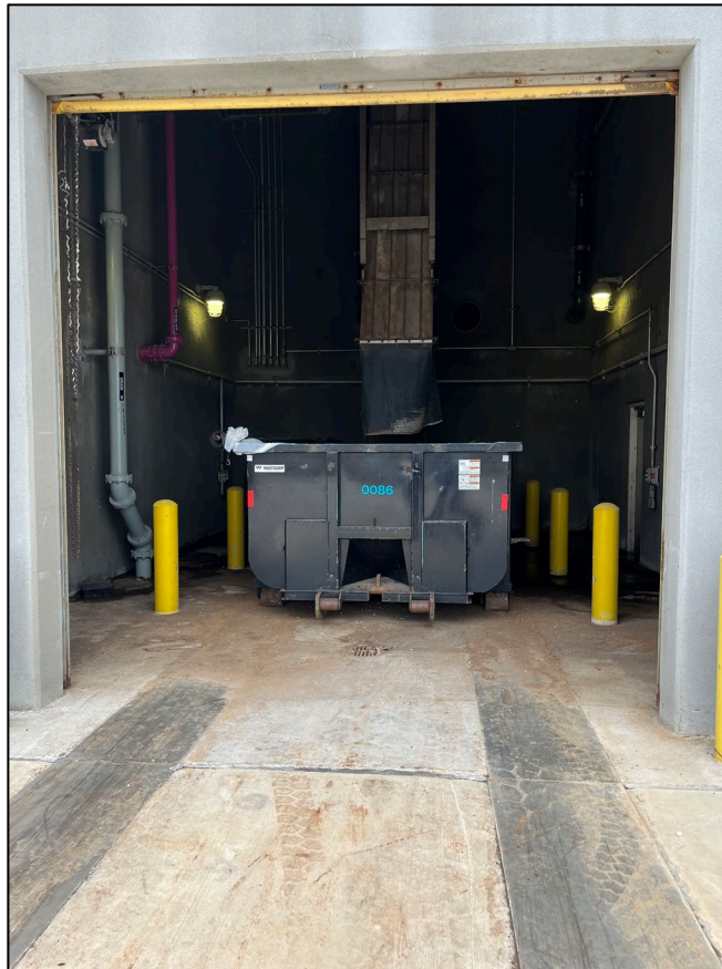
22. Photo taken on north side of the headworks facility on the east side of the subject property facing southwest. A dumpster for collecting large objects and solids from the wastewater influent can be seen. A floor drain that drains back to the wastewater system is visible.
