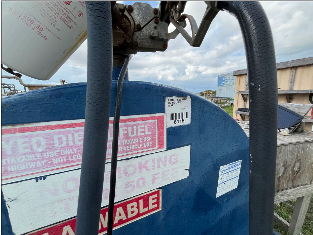
31. Labels on the diesel tank from the previous photo are shown. The tank appears to contain dyed diesel fuel. One label identifies the tank as being double-walled.
