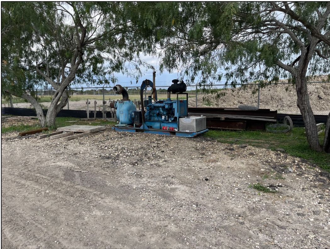
50. Photo taken on west side of subject property facing southwest. A spare pump can be seen.
