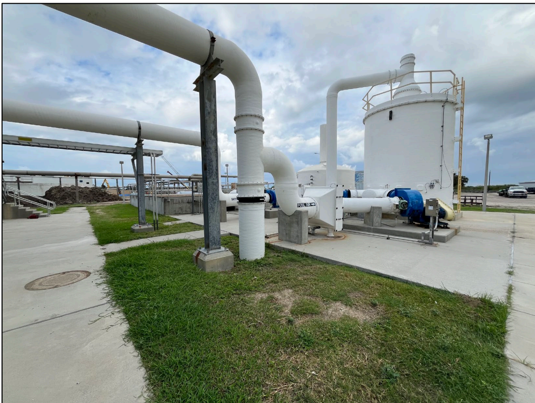
26. Photo taken to west of headworks facility on the east side of the subject property facing southwest. An odor control unit can be seen.
