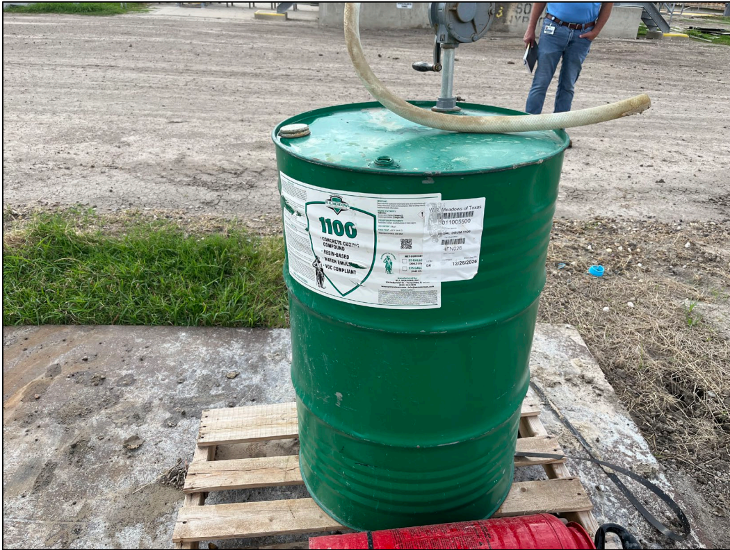
49. Photo taken from west side of subject property. A drum of concrete curing compound can be seen.
