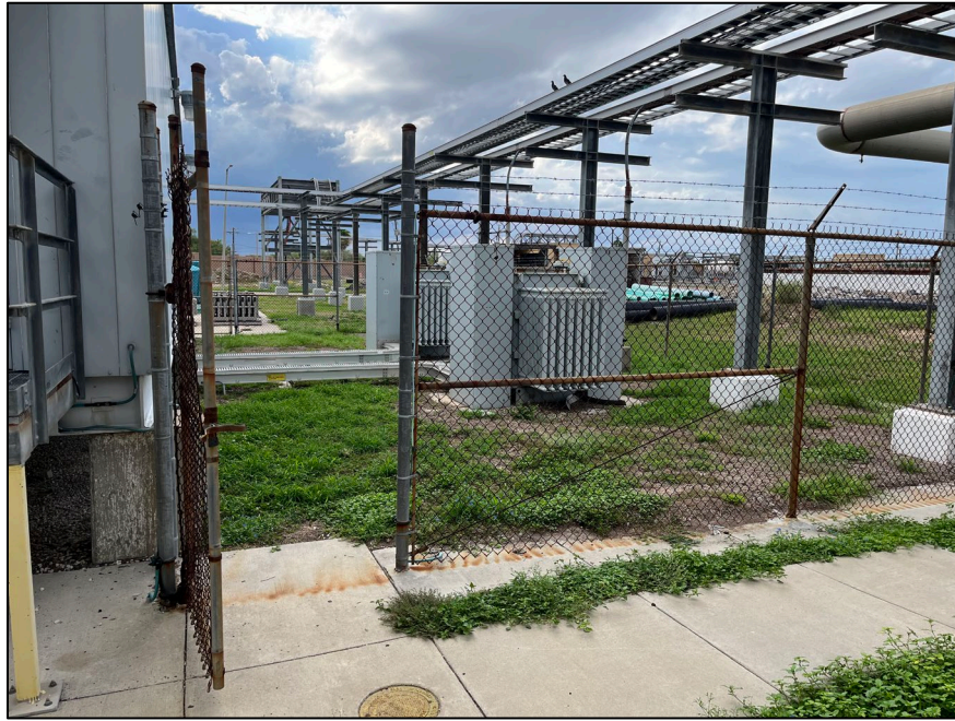
21. Photo taken south of Blower House #4 facing southeast. Two pad-mounted transformers can be seen. No markings were observed to indicate the units are PCB-free.
